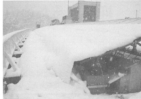
Fig. 5 The snow on PV modules connected it with the snow on the floor
